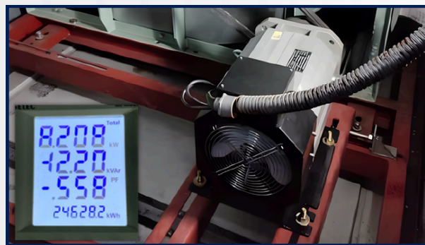
PMSM motor driving an HVAC fan for efficient air circulation.
